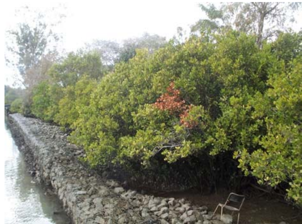
Figure 3. Rock gabions, Brisbane River, placed in front of the mangroves providing protection from erosion.
