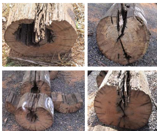
Figure 9 – Purga Creek Girder defects
