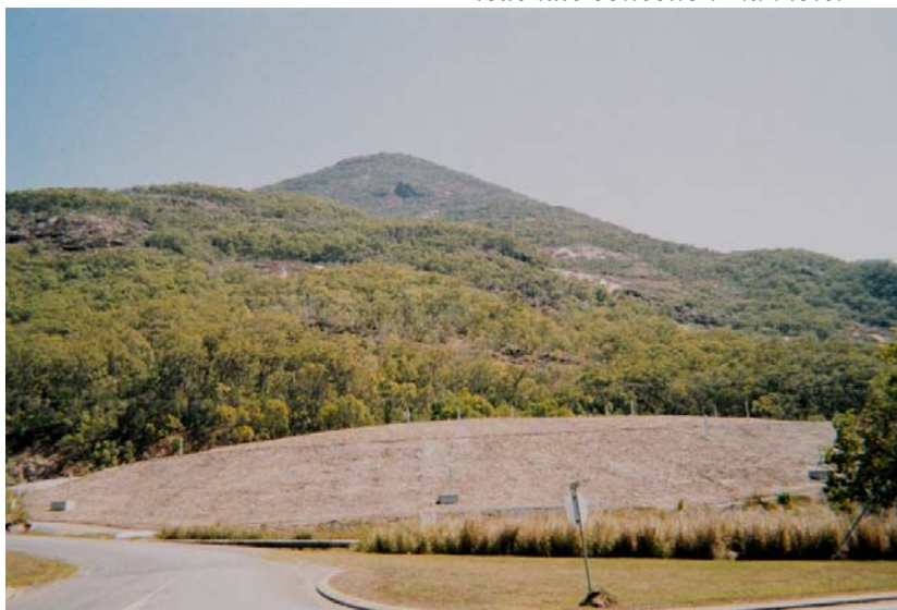
Figures 7 and 8: Deployment of the Geosynthetic Clay Liner (GCL) cap, and sealing around a leachate collection manhole.
