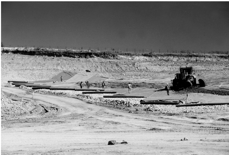
Figure 3: Nonwoven geotextile filter/separator placement - between the leachate collection stone and the waste.
